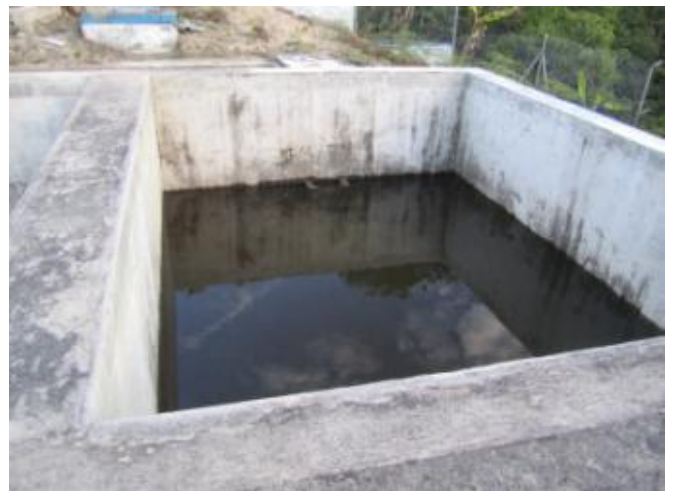
East filter in operation
