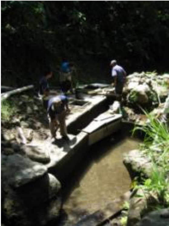
View looking downstream of converging streams at capture tank system. Large tank at bottom of picture is the first settling tank. Water moves from this tank to the long skinny tank in between the first two men, then through the screen and into the covered tank before flowing to the SSF unit.
