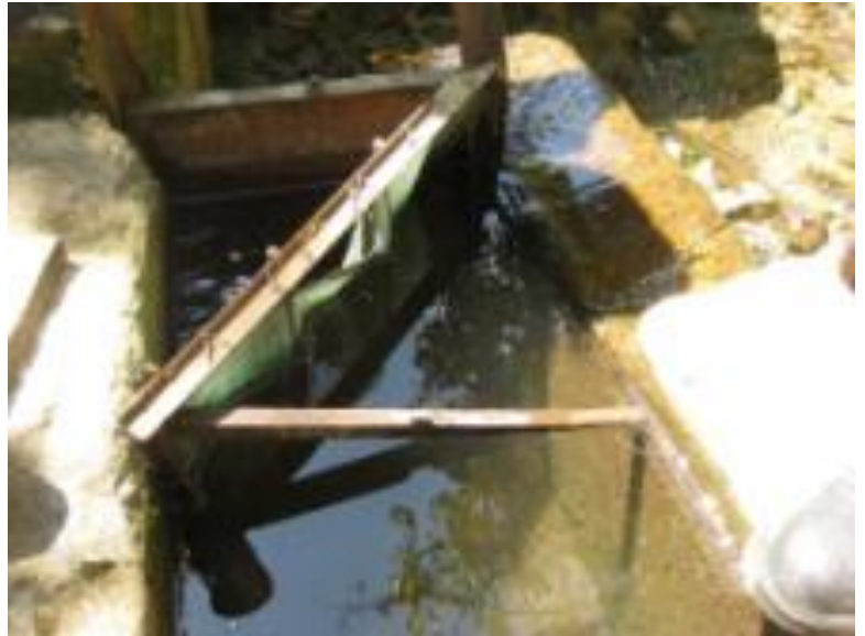
Screen used to remove large debris with space between edge of screen frame and side of enclosed tank allowing for larger particles to pass through.
